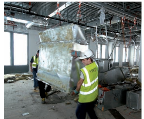
↑ Our £35 million refurbishment of 199 Bishopsgate at Broadgate will deliver 142,000 sq ft of high-quality office accommodation, a BREEAM Excellent rating and 35% better carbon efficiency than current standards – without major façade changes.
