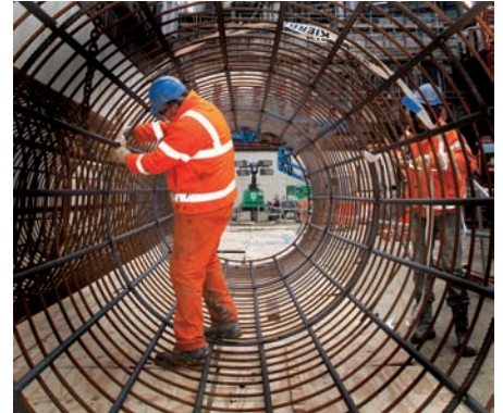
↑ As part of the tender process for The Leadenhall Building, we are evaluating how potential contractors propose to manage environmental and social issues, making sure that this 47-storey tower meets our stringent sustainability standards.
