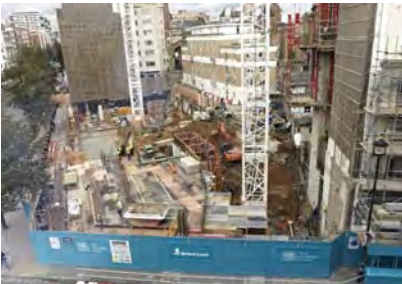
Students got a bird's eye view of the construction site for Marble Arch House from British Land's Head Office, York House.
