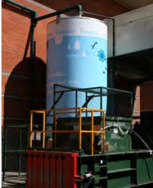
One of four enormous rainwater tanks at Meadowhall.
